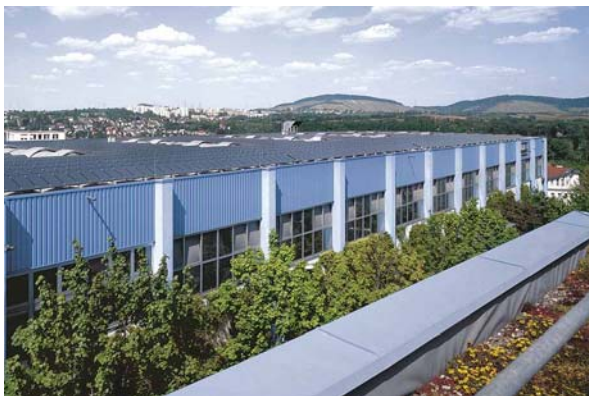
PROFline photovoltaic system with GeneCIS-modules from Würth Solar (Source: Würth Solar)
